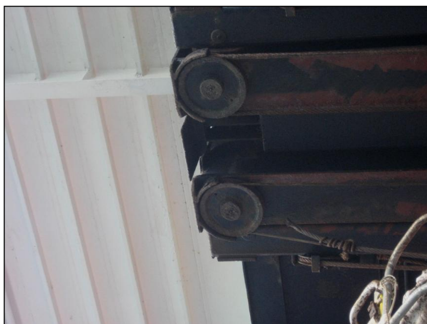
Figure 5: Parted wire rope at its approximate location prior to the accident
