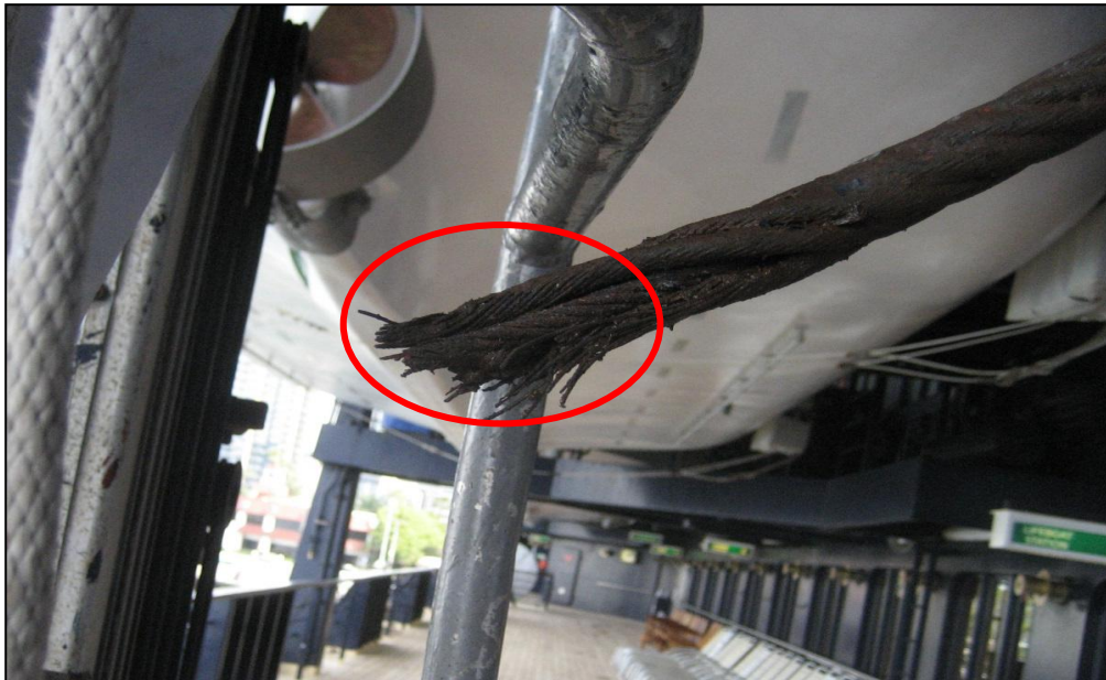
Figure 4: The parted wire rope
